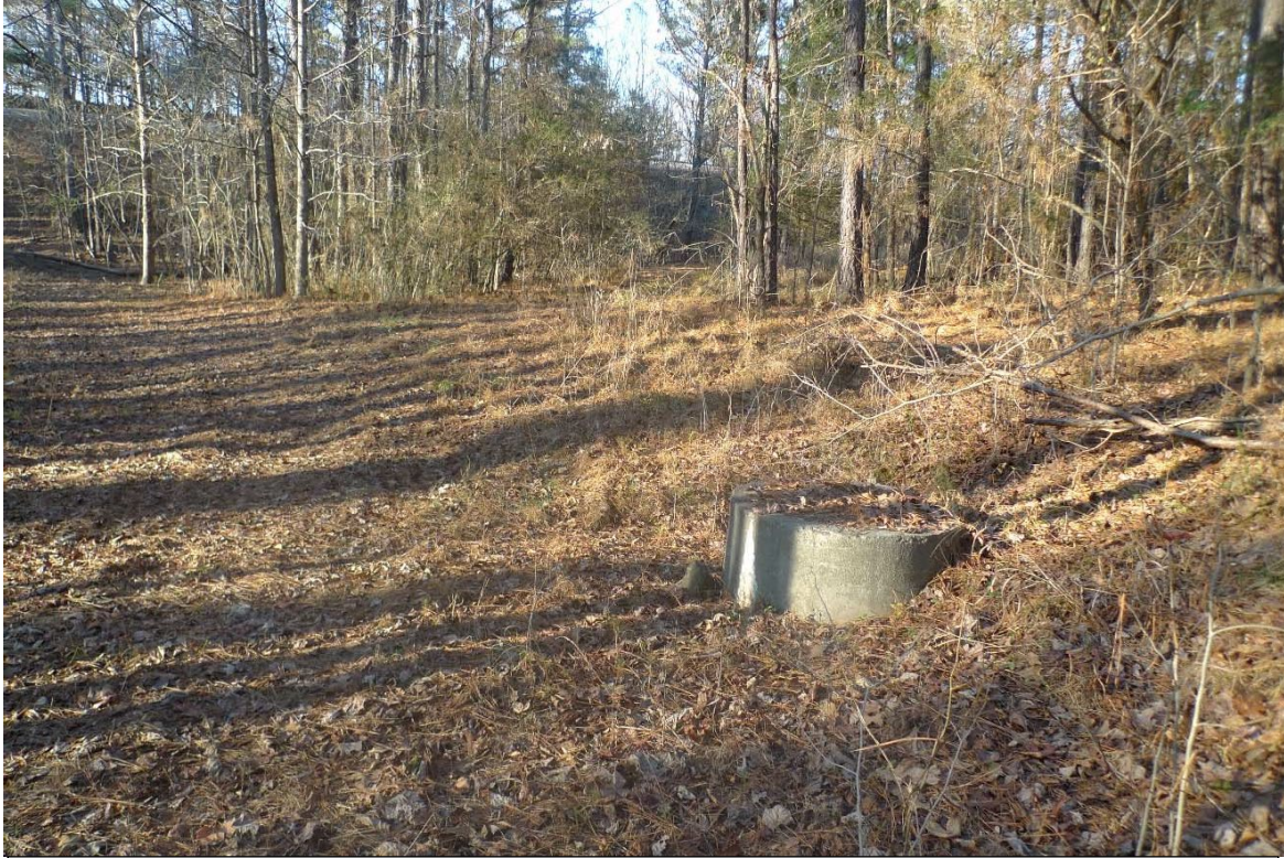
View of sewer line facing south toward the railroad right of way.
